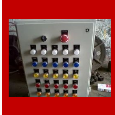
Cranes Control Panel
